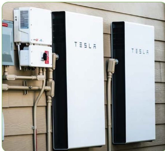
Tesla Powerwall battery system (source: www.ecoaffect.org )
