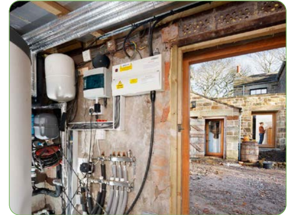
Interior of the outhouse at Hoggerstone Hill Farm, North Yorkshire, showing the ground source heat pump mechanics, with a view towards the converted farmhouse (Source: Adapting Historic Buildings for Energy and Carbon Efficiency - Historic England )
