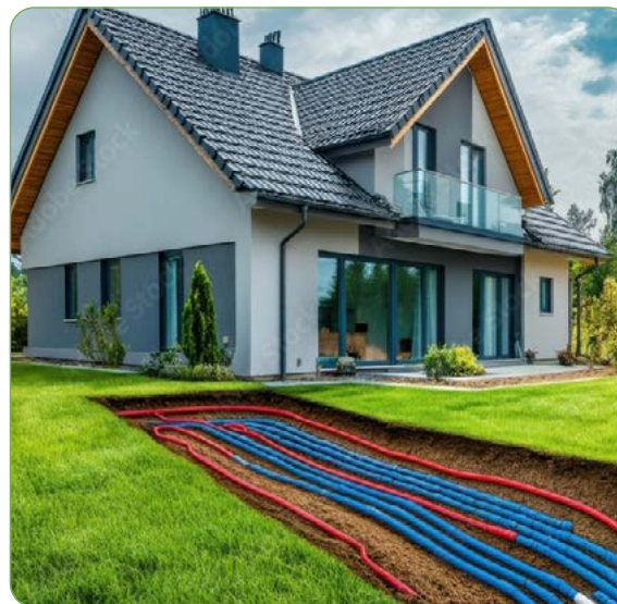
Pipe loop serving a Ground Source Heat Pump
