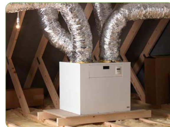
Typical domestic MVHR system fitted in the roof space (source: https://sgs-energy.co.uk ).
